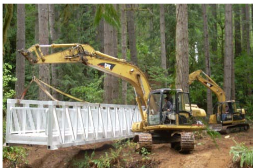
DNR Heavy Equipment Crew puts the new bridge in place across Waddle Creek.
