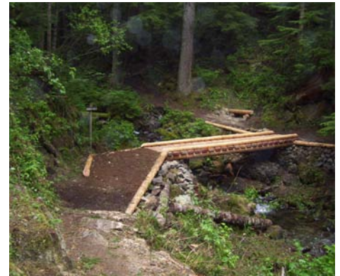
New planking was added to the bridge near hidden falls on the Tarbell Trail. Photo: DNR/Tim Walker
