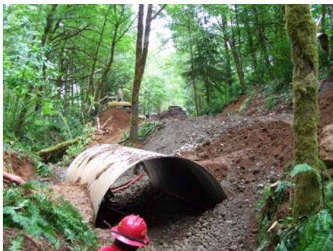
The new Culvert being placed by DNR Heavy Equipment and Cedar Creek Correctional Crews for the Green Line #6 Trail in Capitol Forest Photo: DNR/Nick Cronquist
